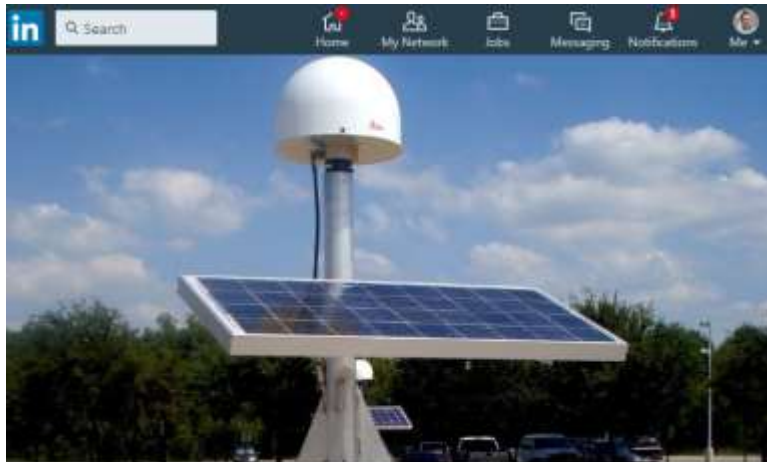
Photo showing a solar powered CORS. Image courtesy of wikipedia
